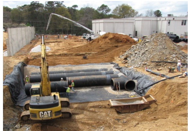
The storm water detention system at LaGrange High School was custom-tailored using large diameter corrugated HDPE pipe to fit a tight area.
